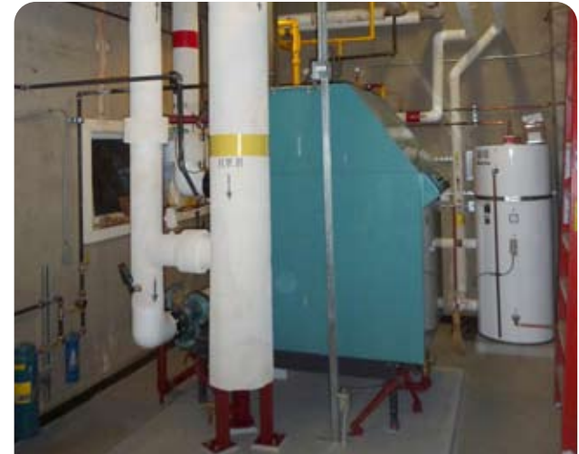
Last year, nine boilers were replaced at Renfrew Community Centre, Vancouver Aquatic Centre, Sunset Arena, Hastings Community Centre and Sunset Nursery.
