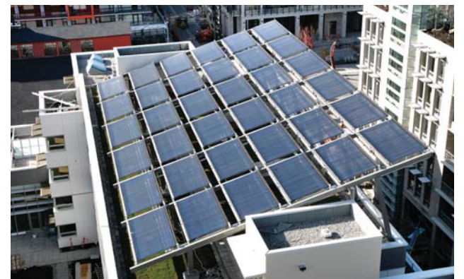
Solar array and green roof atop the Net Zero building.
