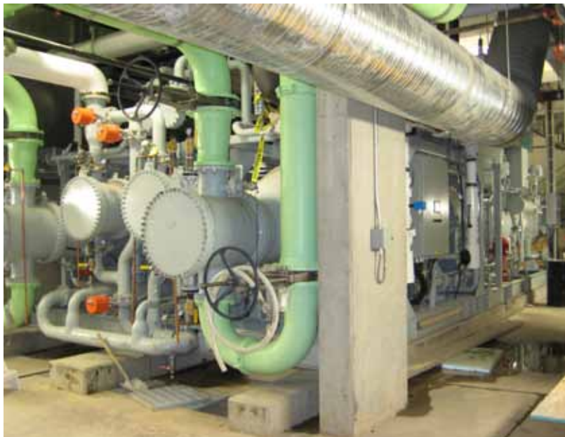
Similar to a geothermal application, heat pumps at the False Creek Energy Centre are used to transfer the heat energy from the wastewater to a hot-water distribution system. In Vancouver, British Columbia, wastewater-heat recovery outperforms geothermal, as the average temperature of wastewater is about 20°C (68°F), which is much warmer than the ground temperature. Kieran McConnell, City of Vancouver, British Columbia
