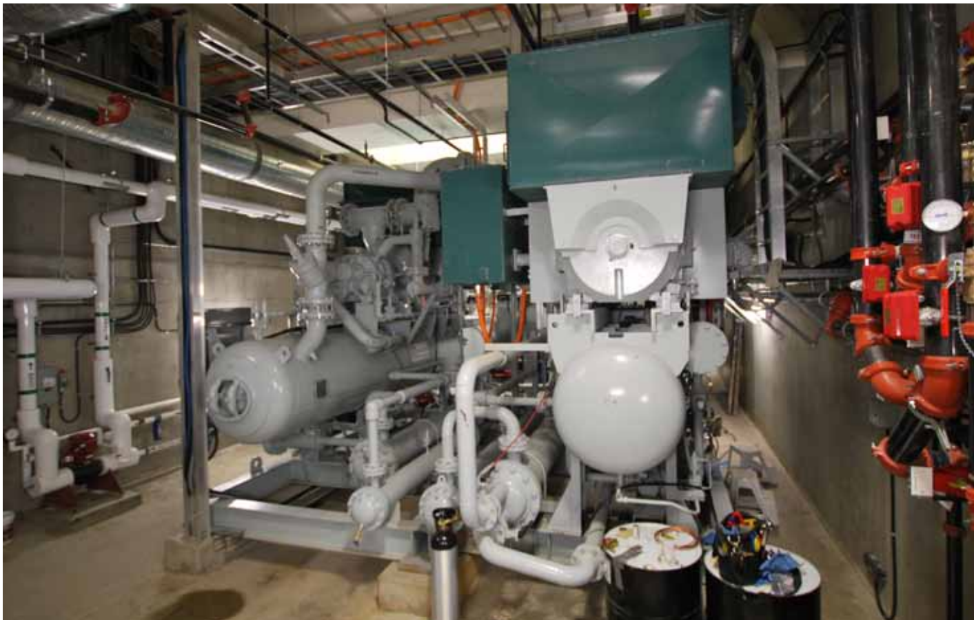
This heat-pump system transfers thermal energy from wastewater to the Neighborhood Energy Utility's thermal distribution system. Kieran McConnell, City of Vancouver, British Columbia
