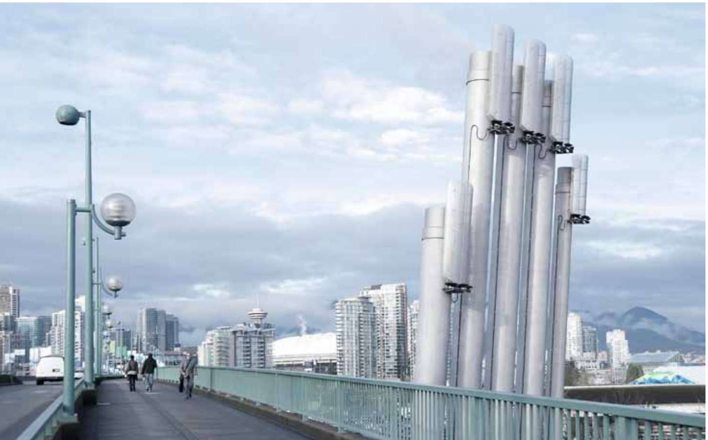
The exhaust stacks of the False Creek Energy Centre blend into the skyline of Vancouver, British Columbia. The energy center, owned and operated by the Neighbourhood Energy Utility, is the first utility in North America to capture and use waste heat recovered from untreated urban wastewater. Ausenco Sandwell
