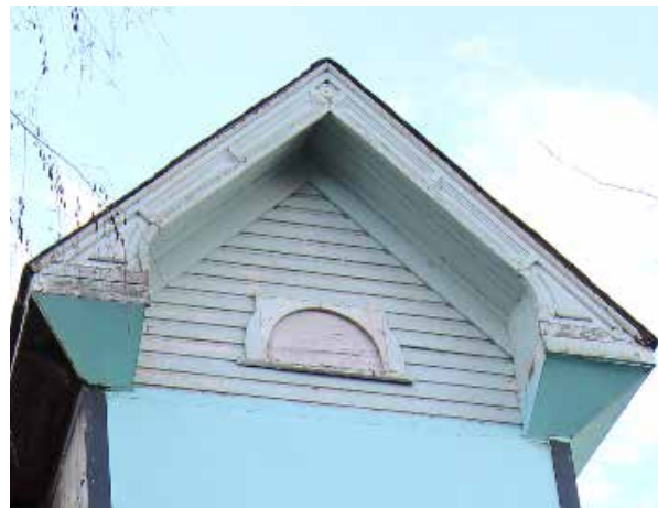
Top: Condition of surviving wood trim and chimney [Donald Luxton & Associates]
