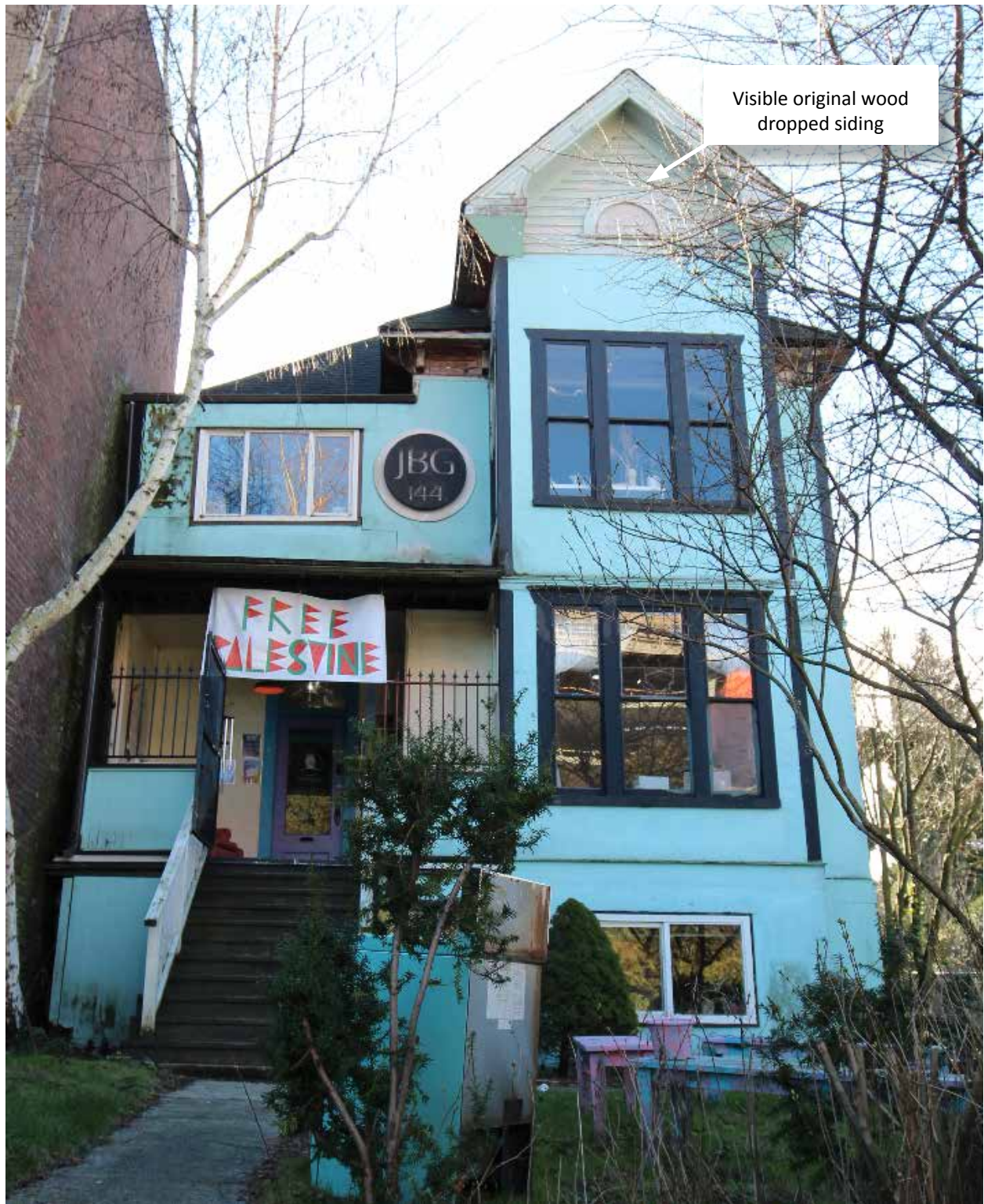
Condition review of front elevation with noted narrow wood dropped siding [Donald Luxton & Associates]
