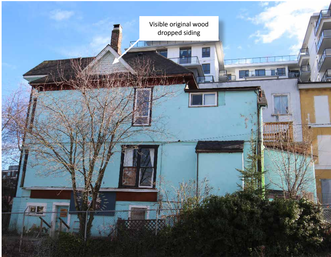
Condition review of side (west) elevation with noted narrow wood dropped siding [Donald Luxton & Associates]
