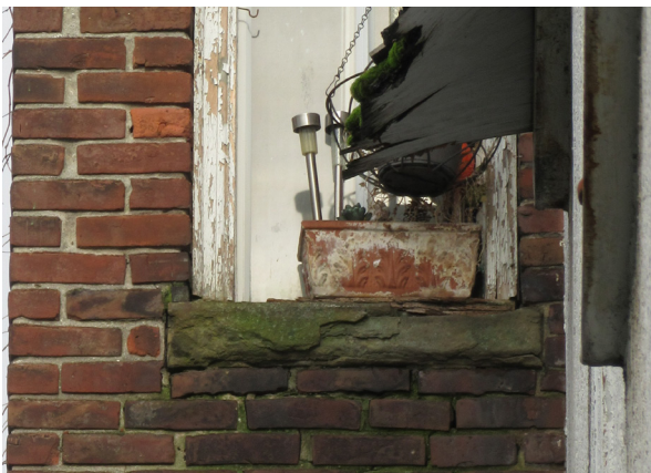
Masonry deterioration at sill on rear elevation window.
