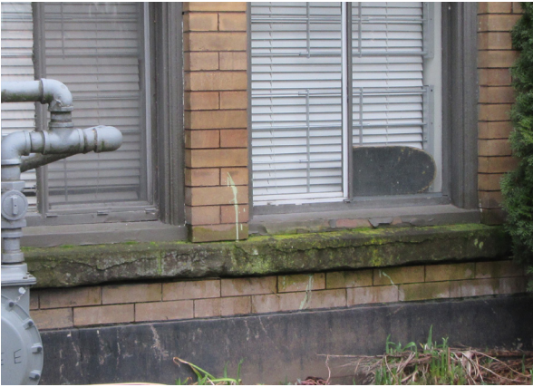
Sill deterioration under north elevation window.
