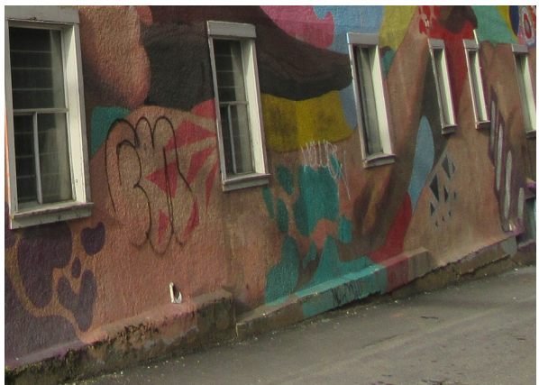
Stuccoed east elevation showing large ledge along top of foundation. Possibility that brick was also present on east elevation due to presence of sill, however, no concrete archival evidence has been found that shows this.
