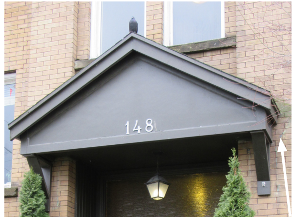
Wood gabled canopy over main entrance. Note outline (white arrow) of previous canopy is evident on the existing brick.
