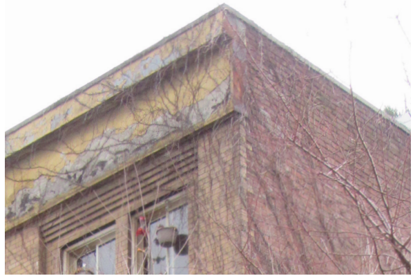
North of parapet has been covered, potentially concealing evidence of original cornice.
