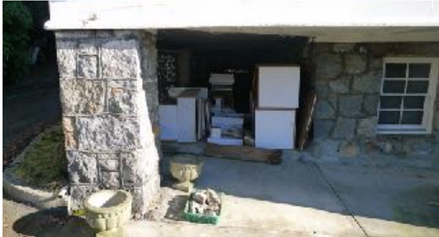
The stone piers and basement foundation showing the standing seam mortar joints
