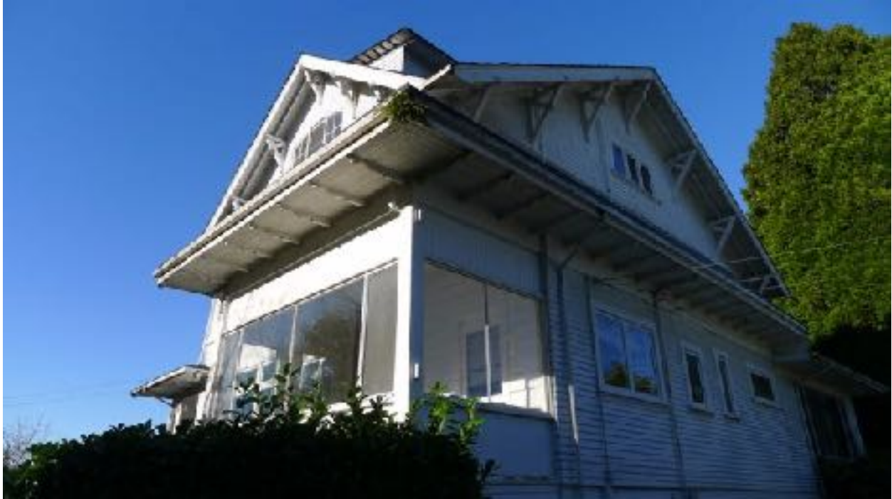
East and south side of the house with kitchen porch showing the addition of a dormer on the side gable.
