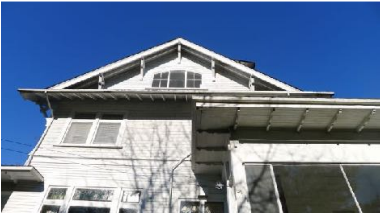
South side of the house with kitchen porch showing the closed in sleeping porch.
