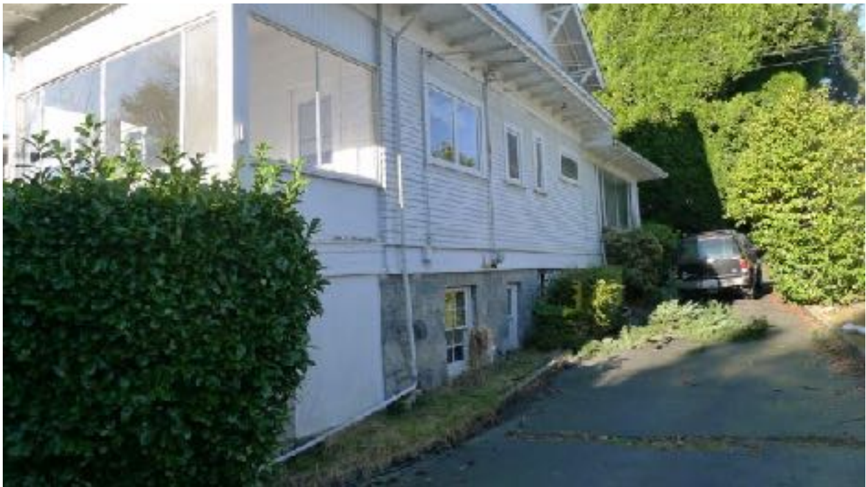
East side of the house looking from the kitchen porch showing the granite foundation
