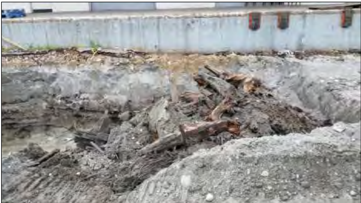
Photograph 2: View of the fill material quality and wood content – looking east. June 1, 2015.
