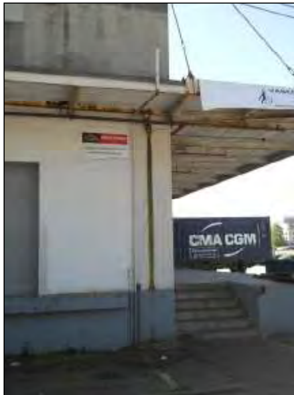
Photograph 8: A cut-off metal pipe observed on the northwest portion of 456 Prior Street (looking south)
