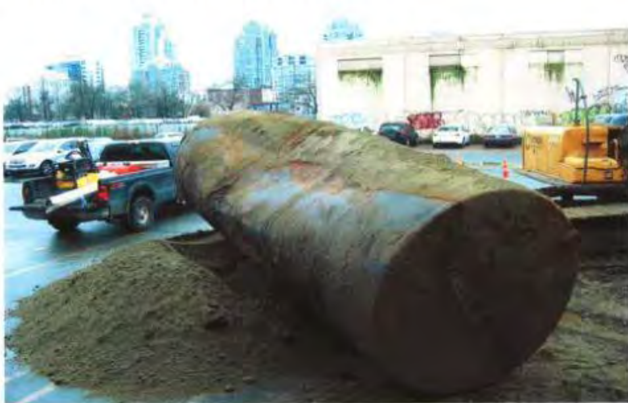
Photo 2 – Fuel storage tank after removal from ground. 5.3 m long by 1.5 m diameter
