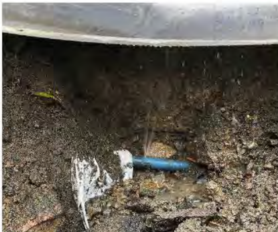
Photo 2: Water connection leak – March 25, 2019
