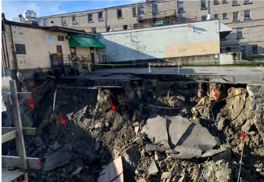
Photo 21: Post failure, visible anchors remain secured
