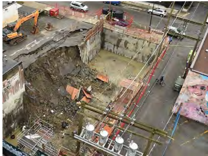
Photo 10: Aerial view of shoring failure (Vancouver is Awesome, February 4, 2020)
