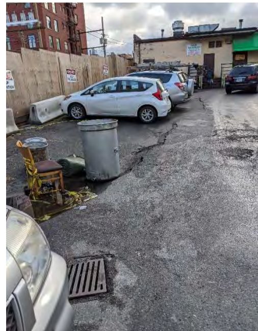
Photo 7: Parking lot cracking, January 28, 2020 (from Prima West)
