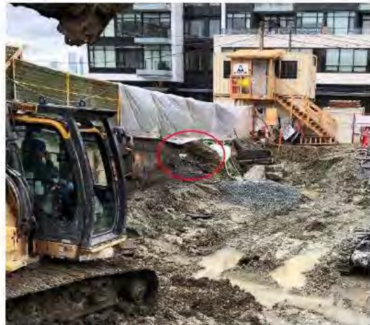
Photo 3: Inferred location of water connection leak March 25, 2019
