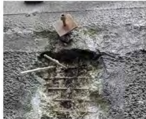
Photo 1: Anchor with loose plate and nut, efflorescence present - January 30, 2020
