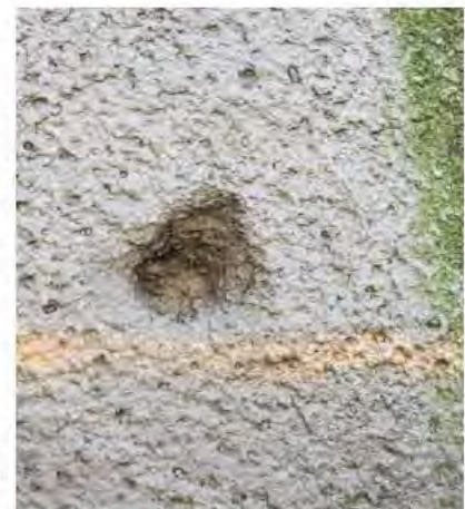
Photo 14: Example of non-functional 'weep hole', South Elevation
