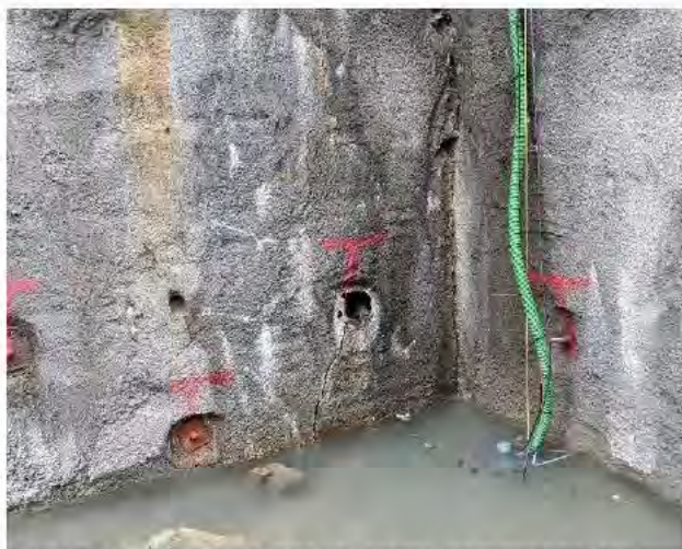
Photo 17: Punched anchors/cracking along West Elevation shoring wall, January 30, 2020
