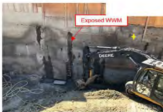
Photo 5: West Elevation Seepage - May 23, 2019
