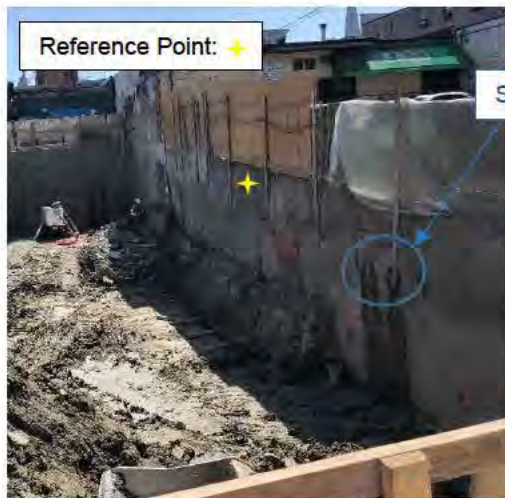
Photo 4A: West Elevation seepage - May 1, 2019
