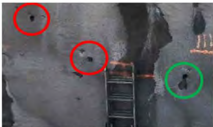
Photo 4: Zoomed Photo 2, showing non functional weepholes versus a weephole showing signs of seepage
