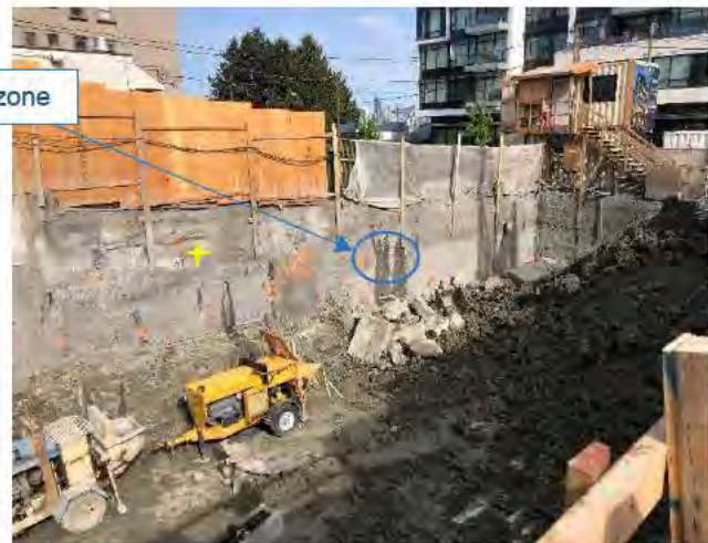
Photo 4B: West Elevation seepage - May 9, 2019
