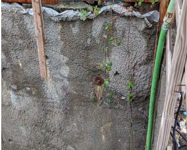
Photo 8: Cracking in the West Elevation, north end (Prima West, Jan. 27, 2020)
