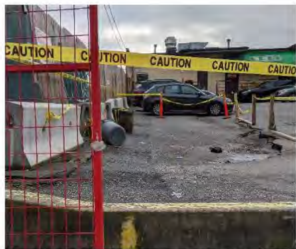
Photo 18: Subsidence of the CNH parking lot, January 30, 2020, January 30, 2020
