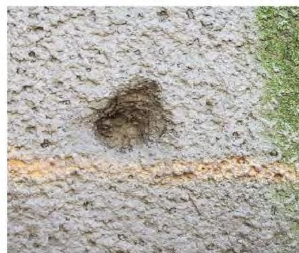
Photo 5: Example of non functional weephole (weephole located on North Elevation)
