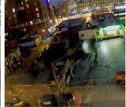
Photo 13: Material retained by existing basement wall collapses, 40 seconds after failure initiation
