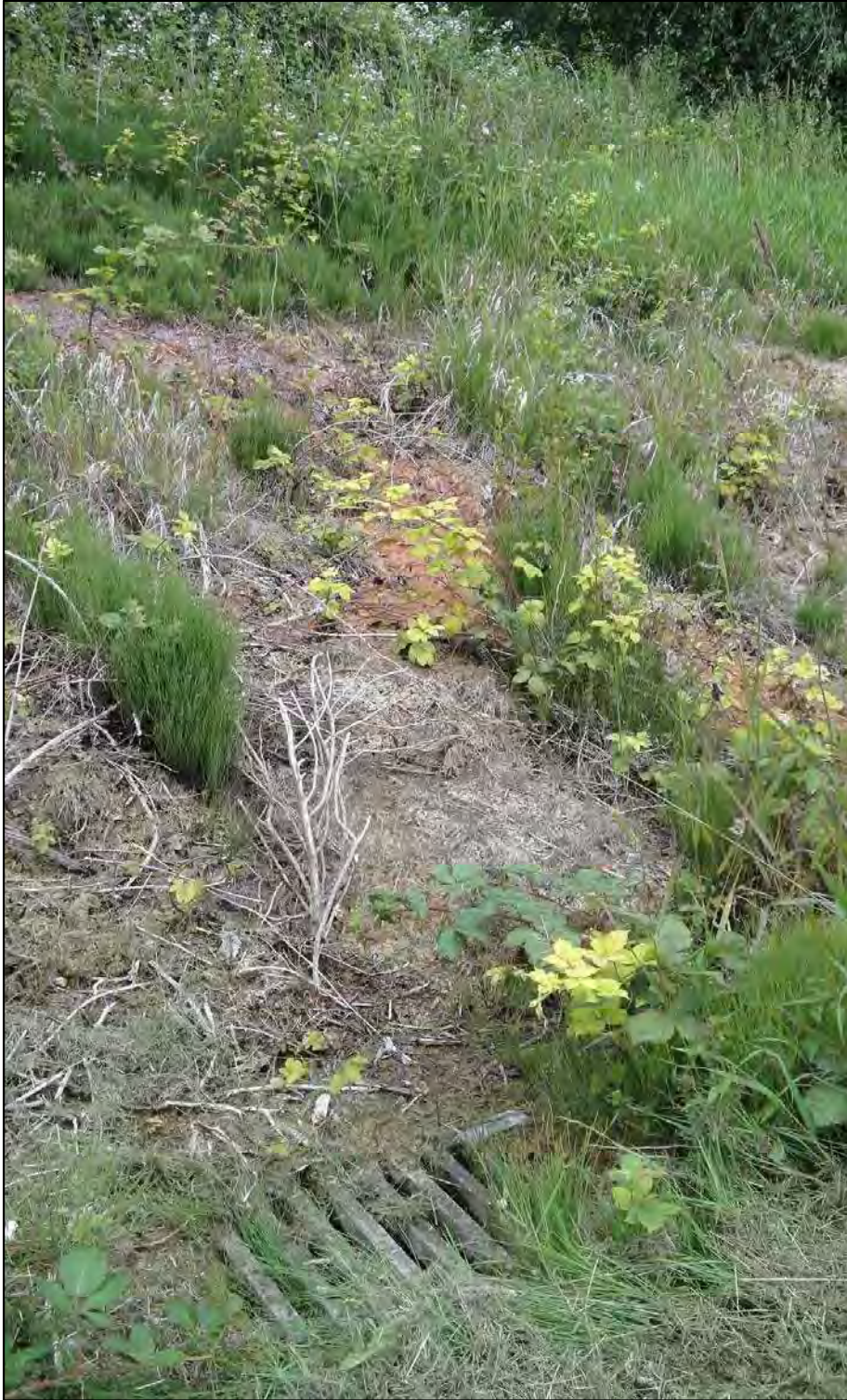
PHOTO 28: Storm sewer catch basin adjacent to iron staining of Seep D. (June 12, 2014)
