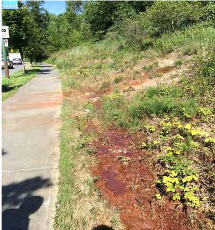
Photo 1: Seepage along south slope 100 m (approx.) east of Kerr St.
