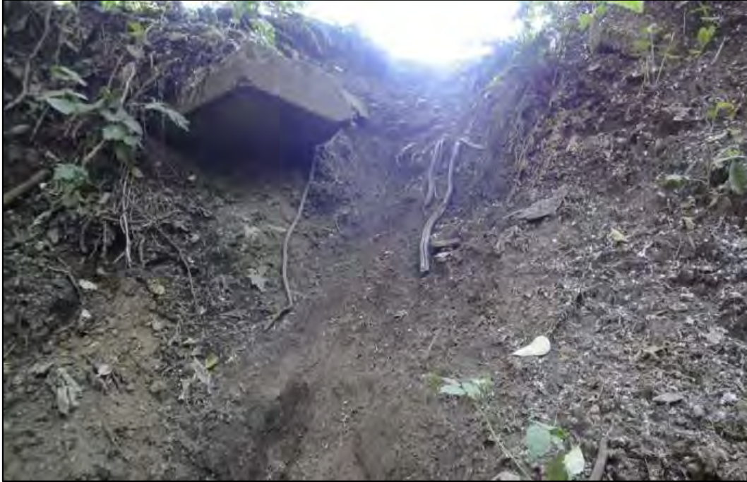
PHOTO 12: Close-up of debris of Photo 11 creek area. (June 12, 2014)
