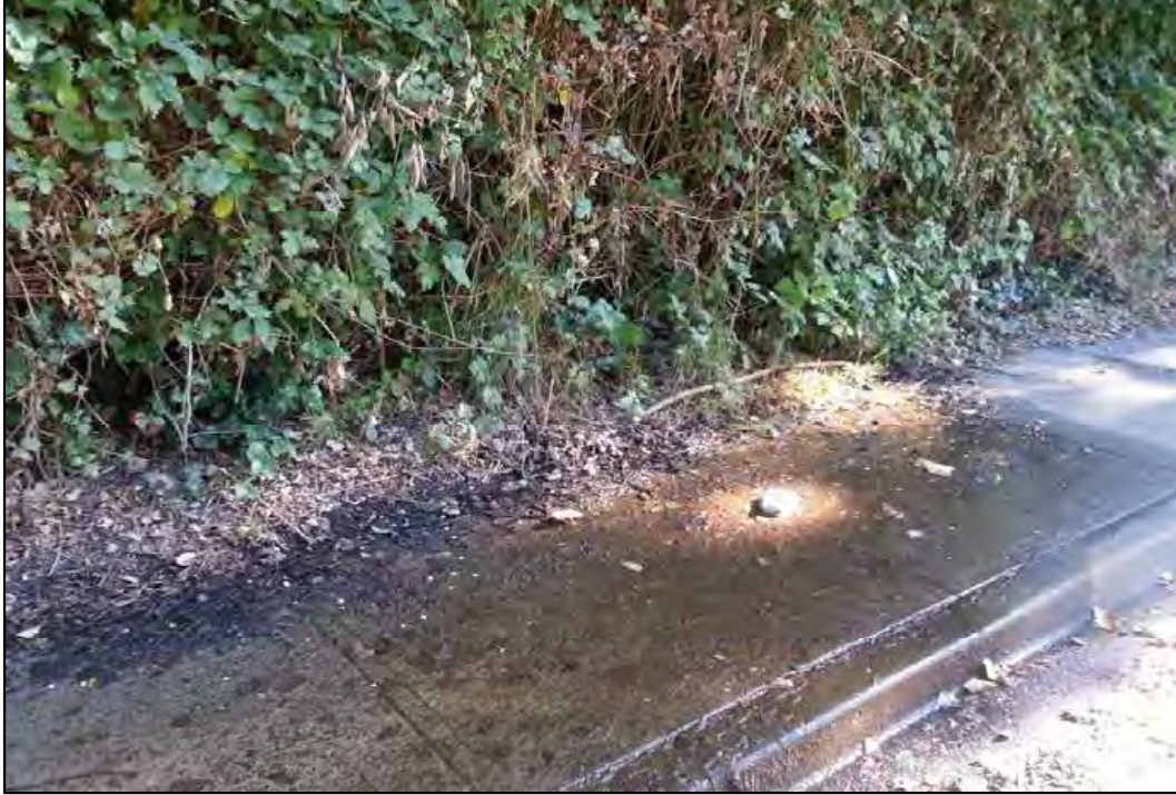
PHOTO 34: Seep onto sidewalk on Matheson Avenue. (June 30, 2014)
