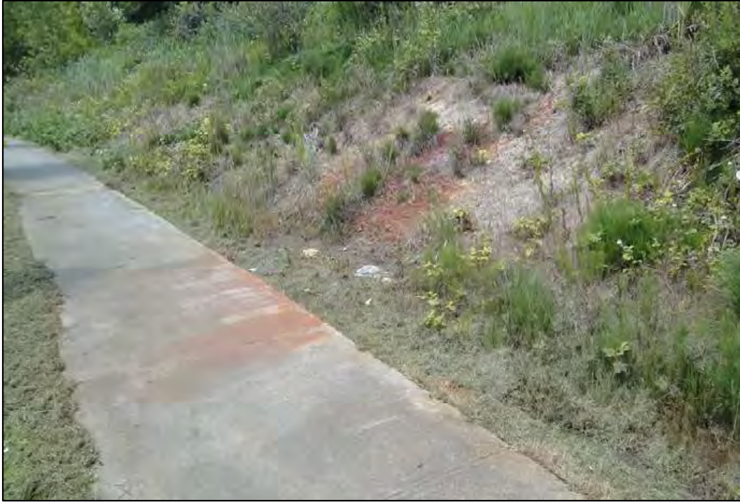
PHOTO 23: Iron staining in seep area (Seep D) along Marine Dr. onto sidewalk. (June 12, 2014)
