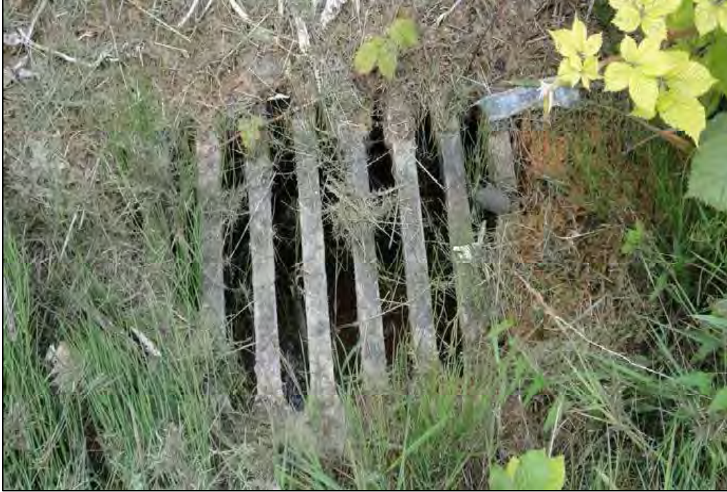
PHOTO 29: Close-up of storm sewer catch basin adjacent to iron staining of Seep D - observed staining discharging into the catch basin and observed within. (June 12, 2014)
