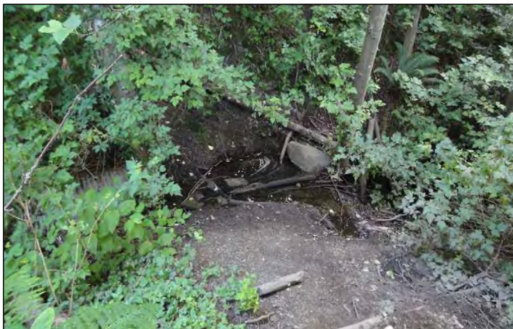
PHOTO 10: New Kinross Creek bank about 100 m north of bridge looking down ravine to creek and culvert within creek. (June 12, 2014)
