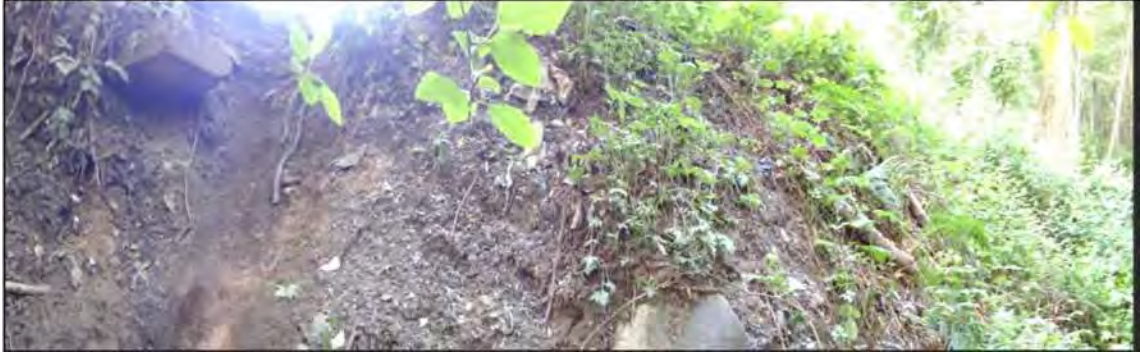
PHOTO 11: Panorama of New Kinross Creek bank about 100 m north of bridge. Exposed debris observed in creek bank (concrete, rubber, glass, shoe, garden hose etc). (June 12, 2014)
