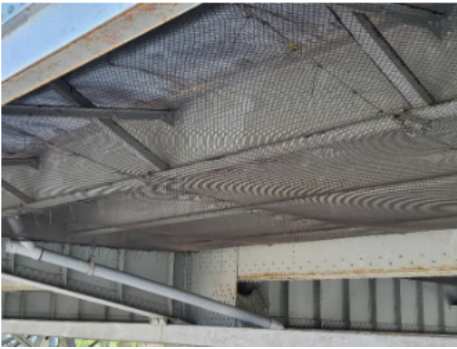
Figure 4 – Debris netting above reported debris location
