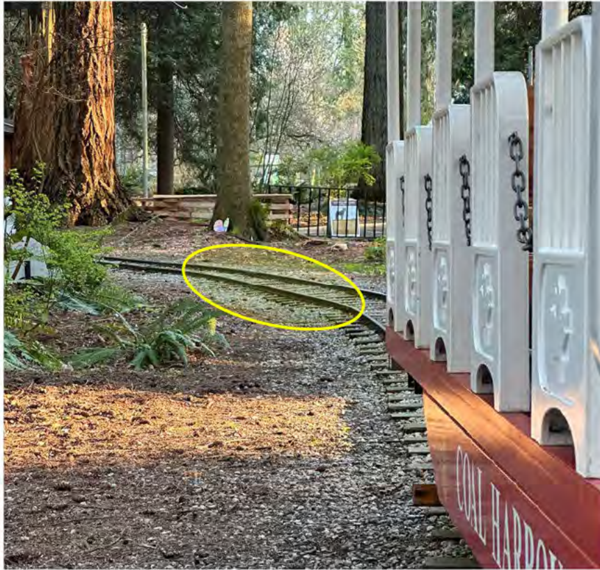
Figure 3 - Depression in Track
