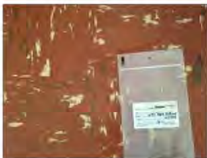
Asbestos-containing vinyl floor tiles.
