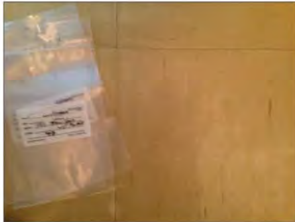
Asbestos-containing vinyl floor tiles.
