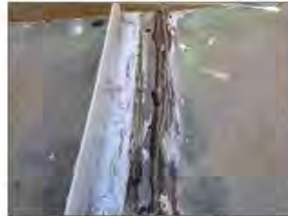
Asbestos-containing silver duct mastic.
