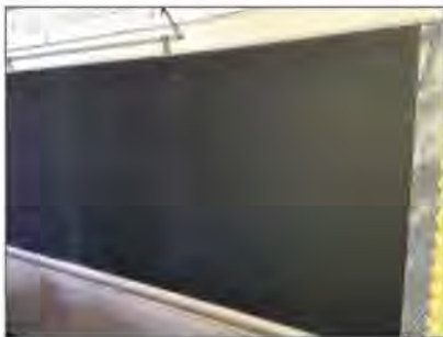
An example of a chalkboard presumed to contain asbestos.
