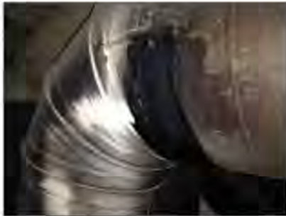
Asbestos-containing black duct mastic.
