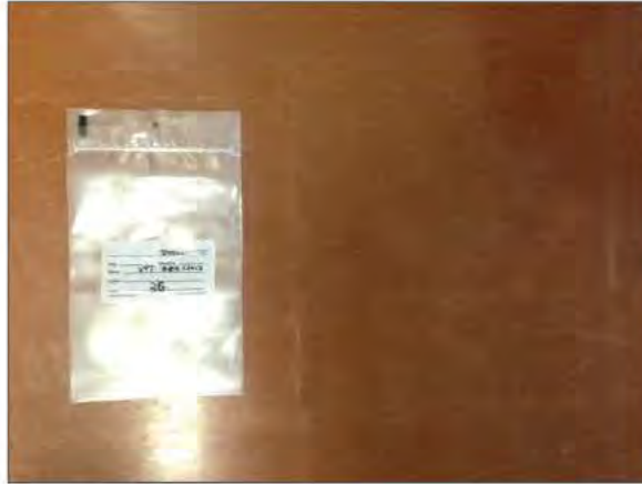
Asbestos-containing vinyl floor tiles.
