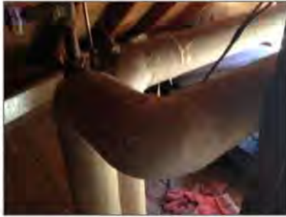
Unlabelled asbestos-containing pipe elbows.
