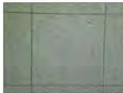
Non asbestos floor tiles concealing asbestos-containing mastic.
