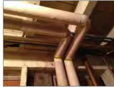
Labelled asbestos-containing pipe elbows.
