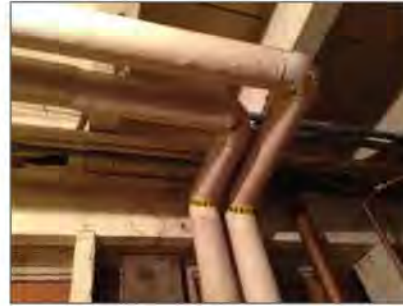
Labelled asbestos-containing pipe elbows.
