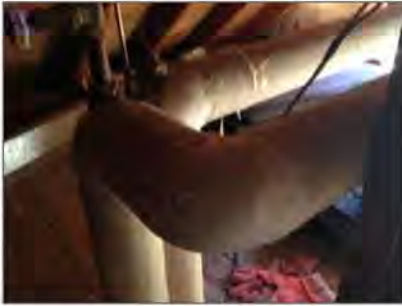
Unlabelled asbestos-containing pipe elbows.
