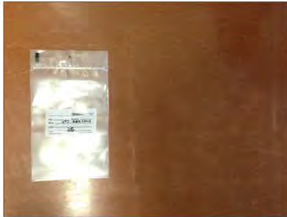
Asbestos-containing vinyl floor tiles.
