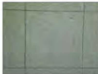
Non asbestos floor tiles concealing asbestos-containing mastic.
