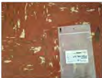
Asbestos-containing vinyl floor tiles.
