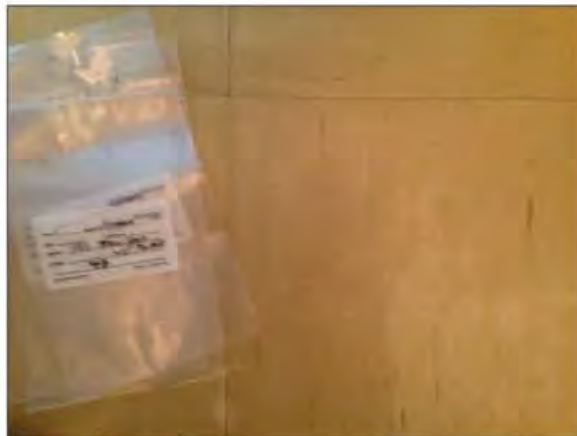
Asbestos-containing vinyl floor tiles.
