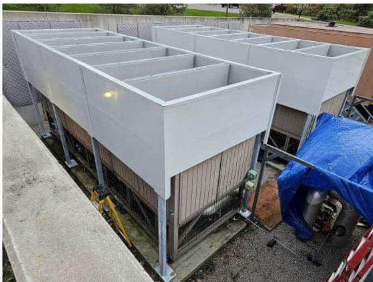
Figure 7: Example installation of a chiller stack on site 6
