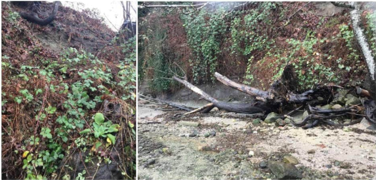
Figure 8: Soil erosion after tree #8 failure (top) and remaining branches (bottom).
