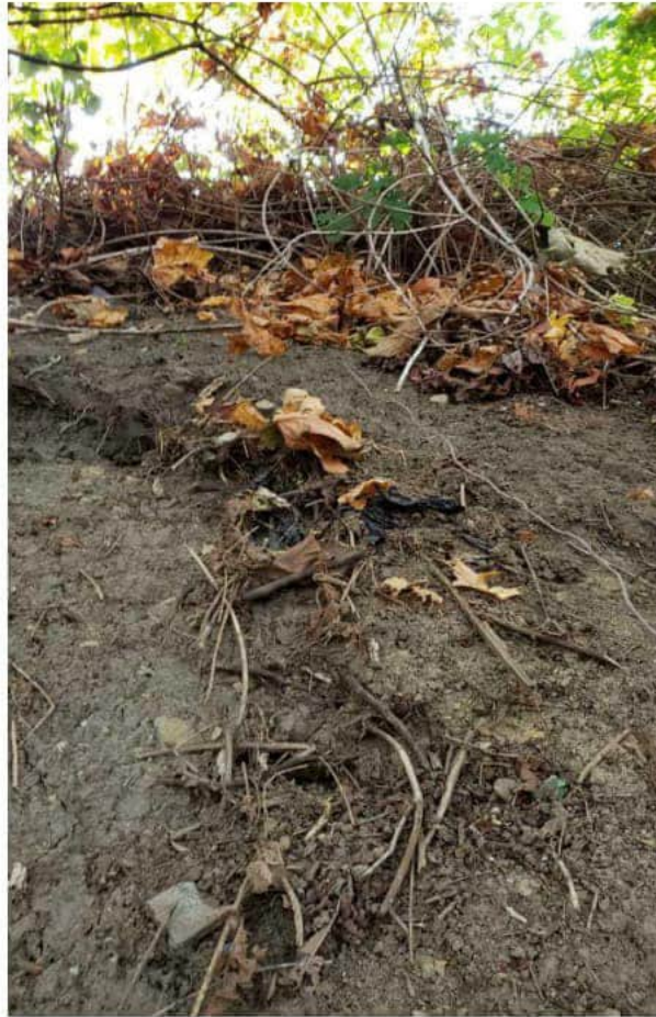
Photograph 5: Inferred fill materials, mixed with debris overlying South Slope
