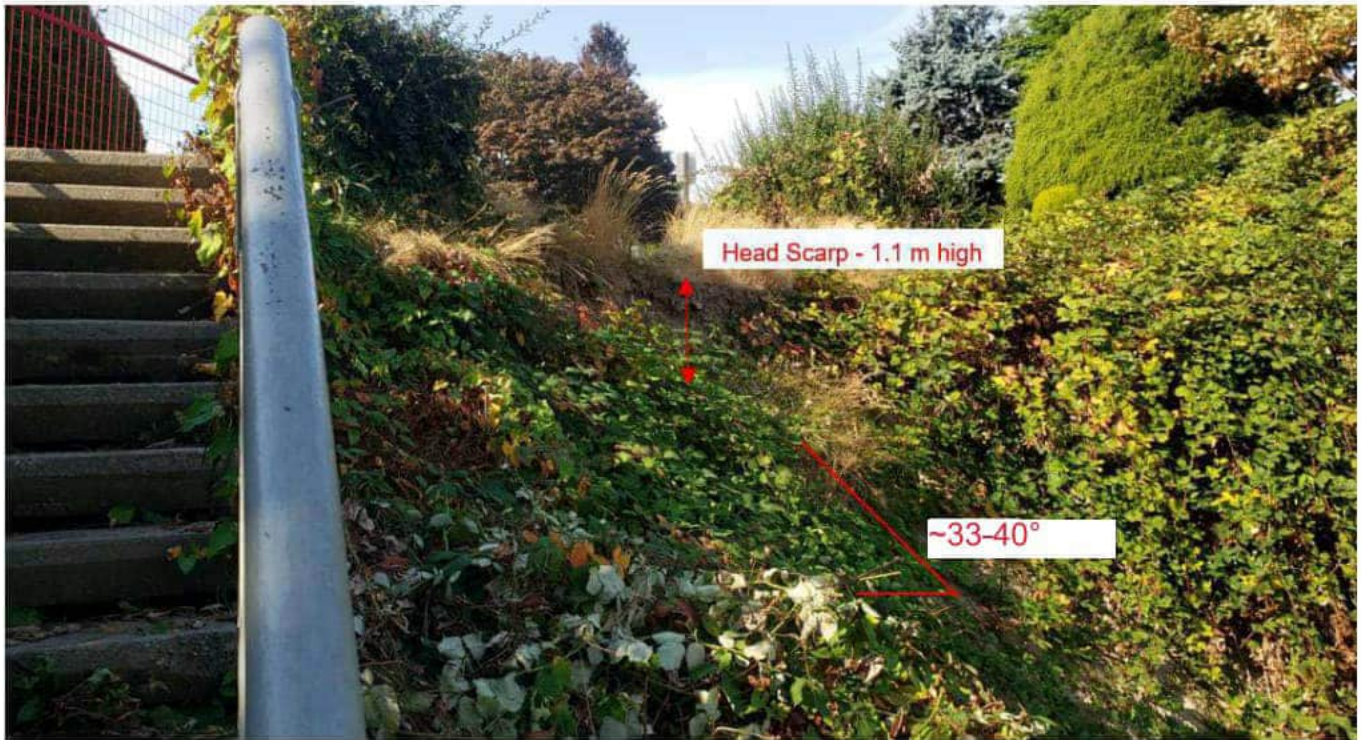
Photograph 1: Headscarp of North Slope (looking North from top of staircase)
