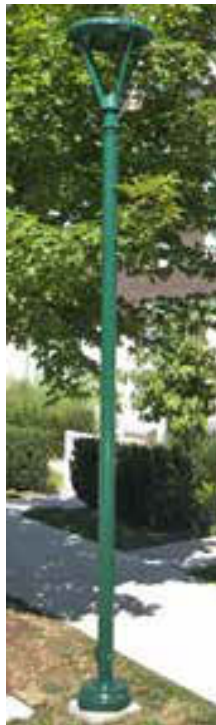
Typical pedestrian standard mounted on pedestrian pole
