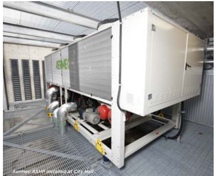
Aermec ASHP installed at City Hall
