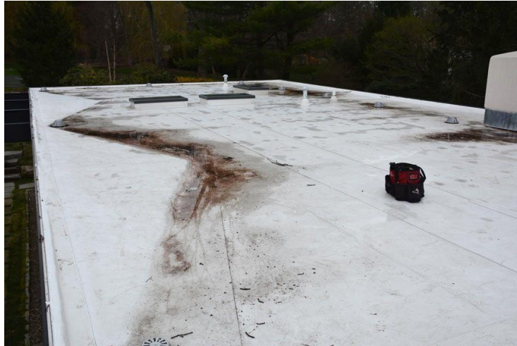
/ Figure 3: Algae growth on cool roof membrane, reducing its solar reflectance. Image source: [11]
