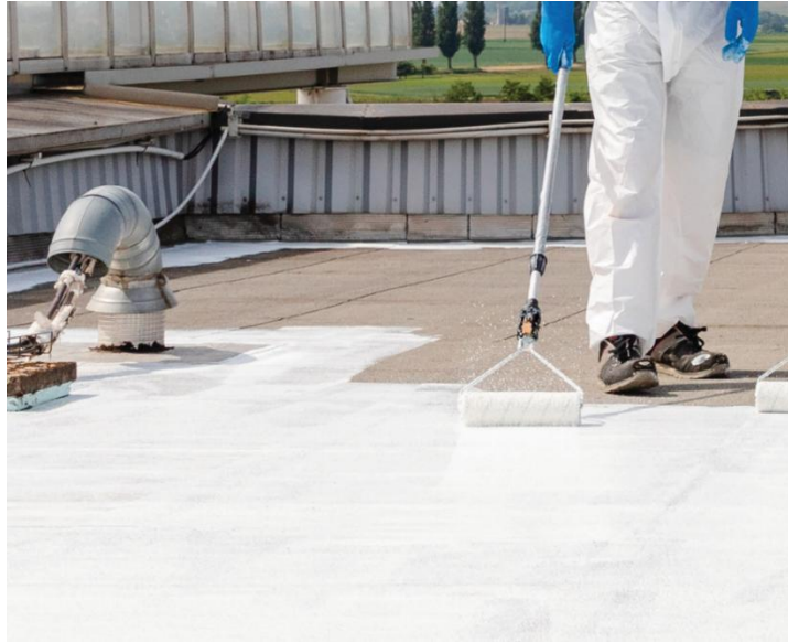
/ Figure 2: Application of a cool roof coating over a modified bitumen membrane. Image source: [4]
