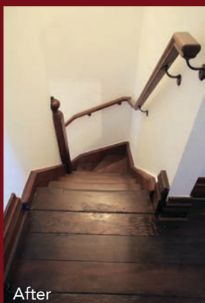
Above: Addressing hazardous stair elements such as missing treads and handrails is a typical requirement under the By-Law. See Section Three for more on stairs.
