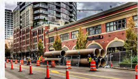
Columbia Street mainline sewer separation in progress. (Photo credit: Dennis Sylvester Hurd via Flickr, CC BY 2.0)
