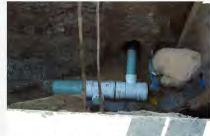
Sanitary sewer replacement and separating/replacing a combined private sewer lateral (Photo Credit: Pam Broviak) 2
