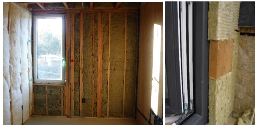
Figure 3: Photo of insulation of batt insulation filling stud cavity without air pockets (left) and over insulation of the window jamb (right).
