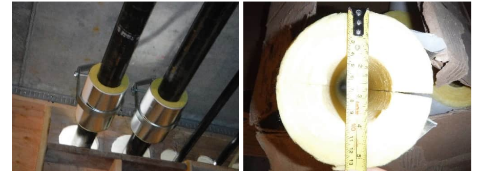
Figure 5: Photo of oversized pipe hangers (left) and documentation of domestic hot water pipe insulation thickness.
