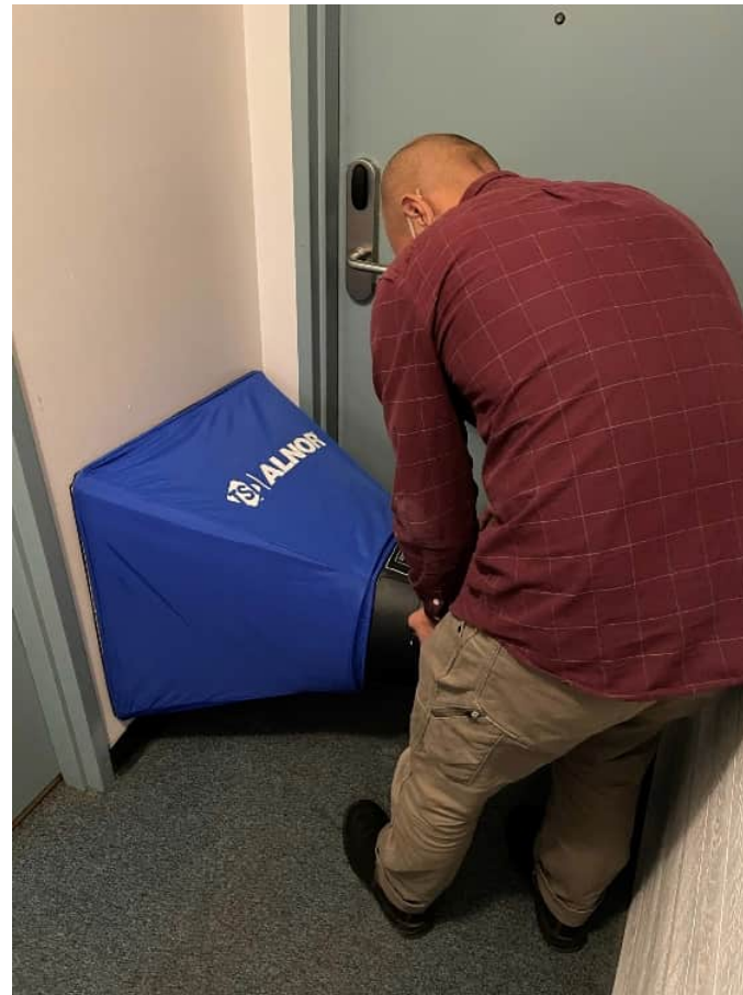
Figure 8: All supply and extract grilles to be adjusted, balanced and recorded at the normal ventilation rate.
