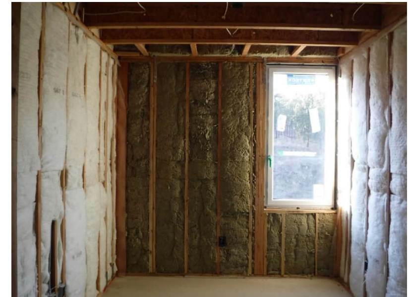
Figure 2: Installation of insulation. Poor installation will result in derating of the as-built PHPP model.
