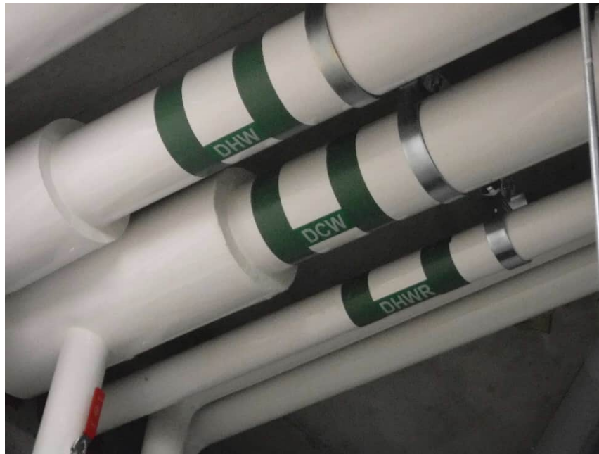
Figure 3: Use of oversized pipe hangers to ensure continuous insulation of service water heating pipes.
