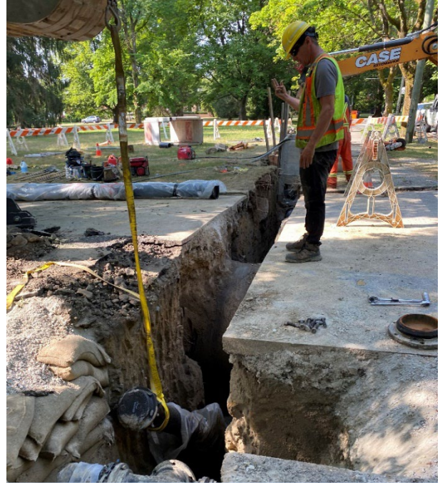
Shaughnessy East: Installing water main “arch” under 1800 mm Metro Vancouver water main.
