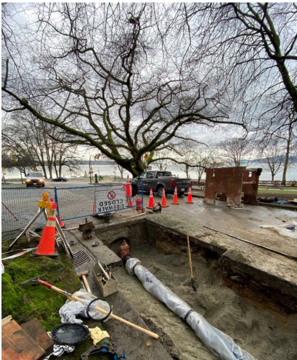
Burnaby Street and Bidwell Street: New water main laid on the south end of Burnaby Street.
