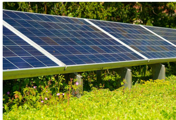
Above - Photo-Voltaic Solar Panels on a Green Roof
