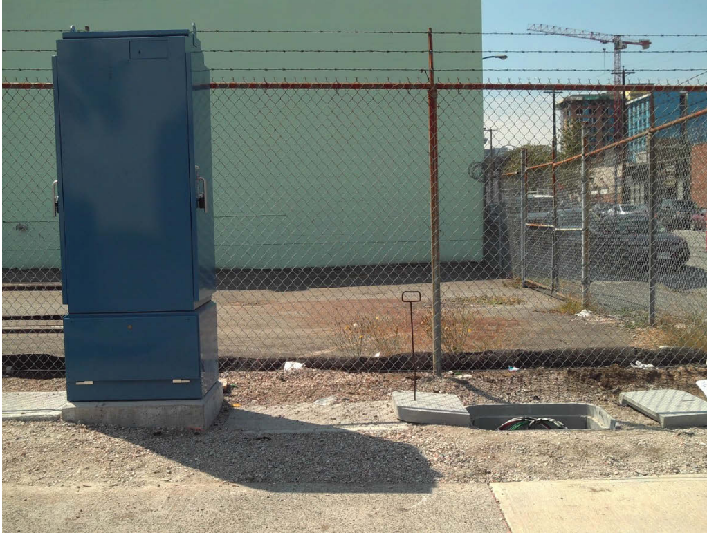
Figure 10-18: Type 332 Controller Cabinet with Battery Box
