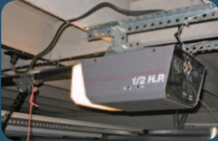
Garage door openers are a common source of noise, which can be reduced by using vibration isolating mounts.
